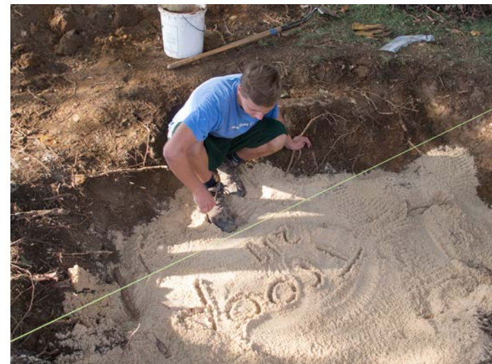
Sand and topsoil were added back to bring the surface to about a foot below grade. Then the surrounding turf grass and soil were removed to create a sloping basin.
