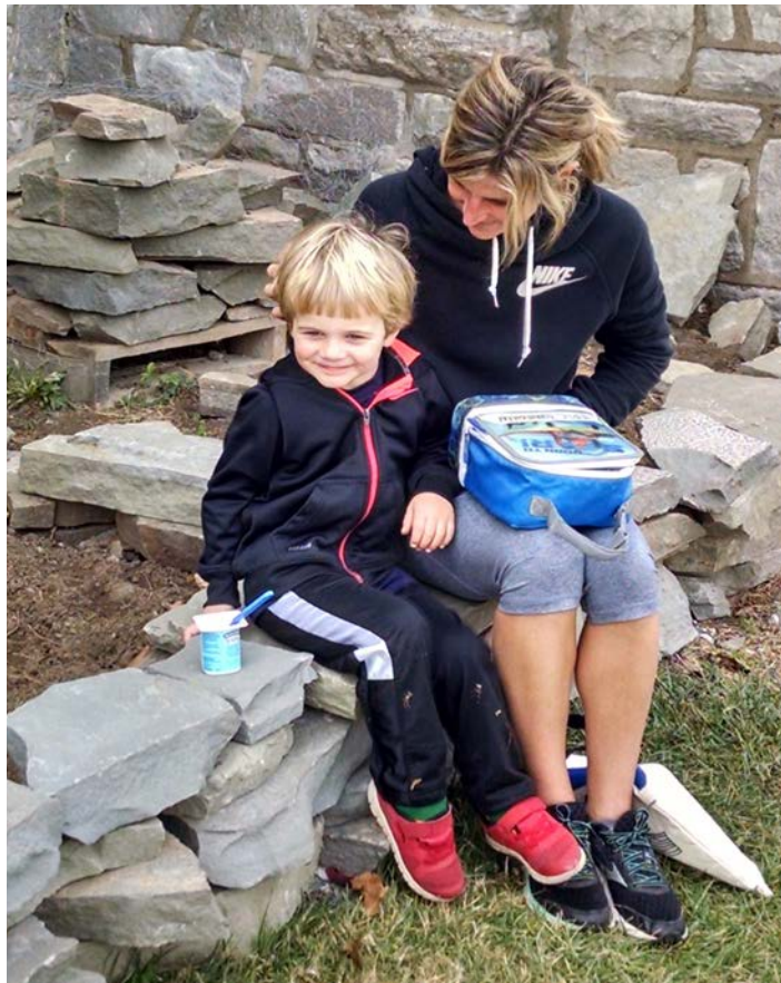
The terraced gardens under construction in October of 2015. Neighbors found it a good place to take a break.
