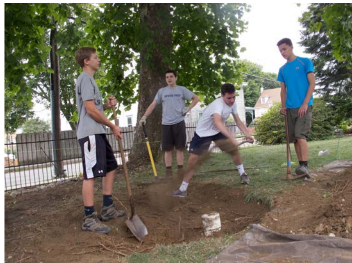
After removing the river rock from the area of the future rain garden, Scouts dug out the center to a depth of about 24 inches, exposing the pipe that carries water from the church roofs.
