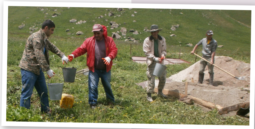
Villagers construct a clean water pipeline thanks to a community development grant.
