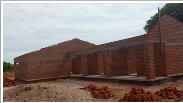
New clinic being constructed at Phalaza. We are so grateful that we have received donations for half of the funds necessary to complete the project and are praying that the remaining funds will soon be provided.
